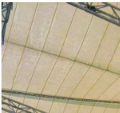
Image 2: Lacquer adhesion problems in translucency. Where lacquer is not performing the coating is directly exposed to soiling and UV attack.
